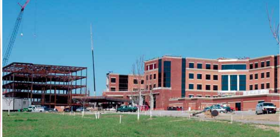
Construction continues toward the December 2007 opening for the new Atrium Medical Center (right) and adjoining professional office building at Premier Health Campus — Middletown.
